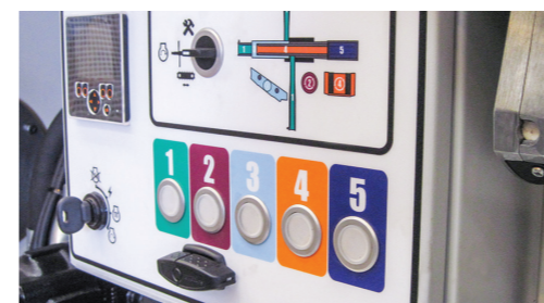
Colour coded control panel for ease of operation
